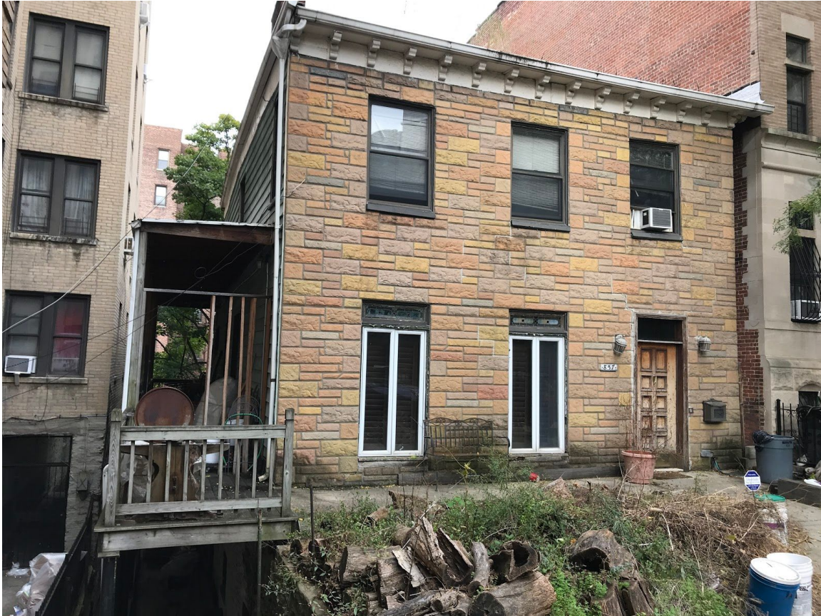
857 Riverside Drive today. The side and rear porches are intact, as is the original clapboard or lapstrake siding, which has been covered in stucco on the front of the house. Photo by URRA
