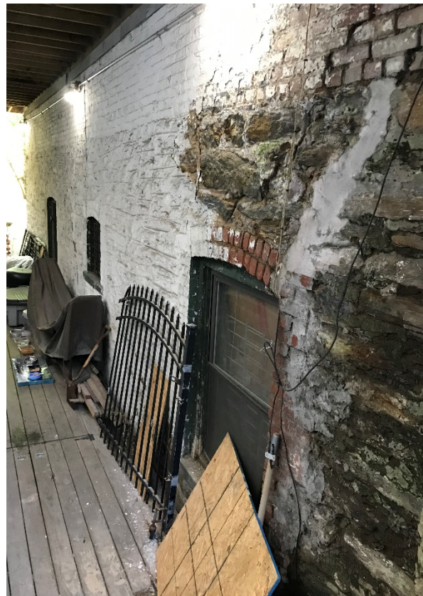
Figure 11 detail of the foundation showing stone and brick coursing and historic windows.
