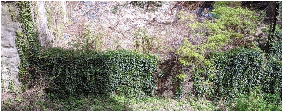
Figure 1: Dry-laid Stone Wall at the Western Edge of the 857 Riverside Drive Property
