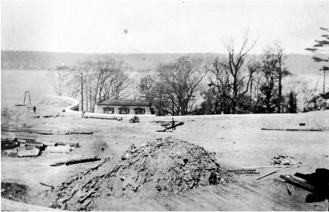
Figure 10: Construction of Riverside Drive at 156th Street, with the Mansard Roof on the Audubon Homestead Barely Visible 48
